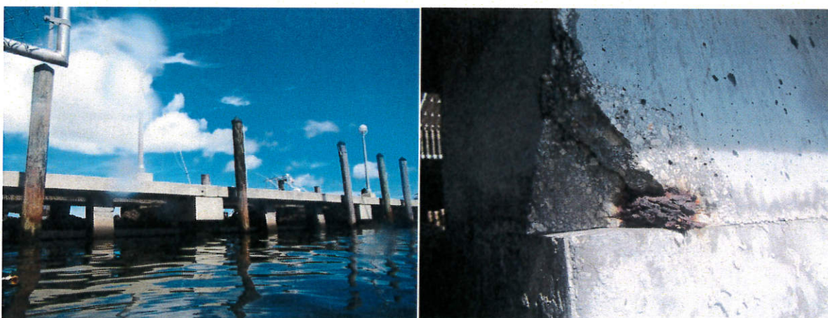
Photo 55: North Concrete Finger Pier (left). Minor concrete deterioration on few piles (right).
