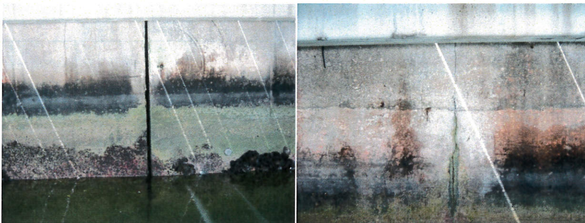
Photo 31: Loss of expansion joint material at expansion joint (left photo) typical. North face of bulkhead exhibited more hairline cracks typical (right photo).
