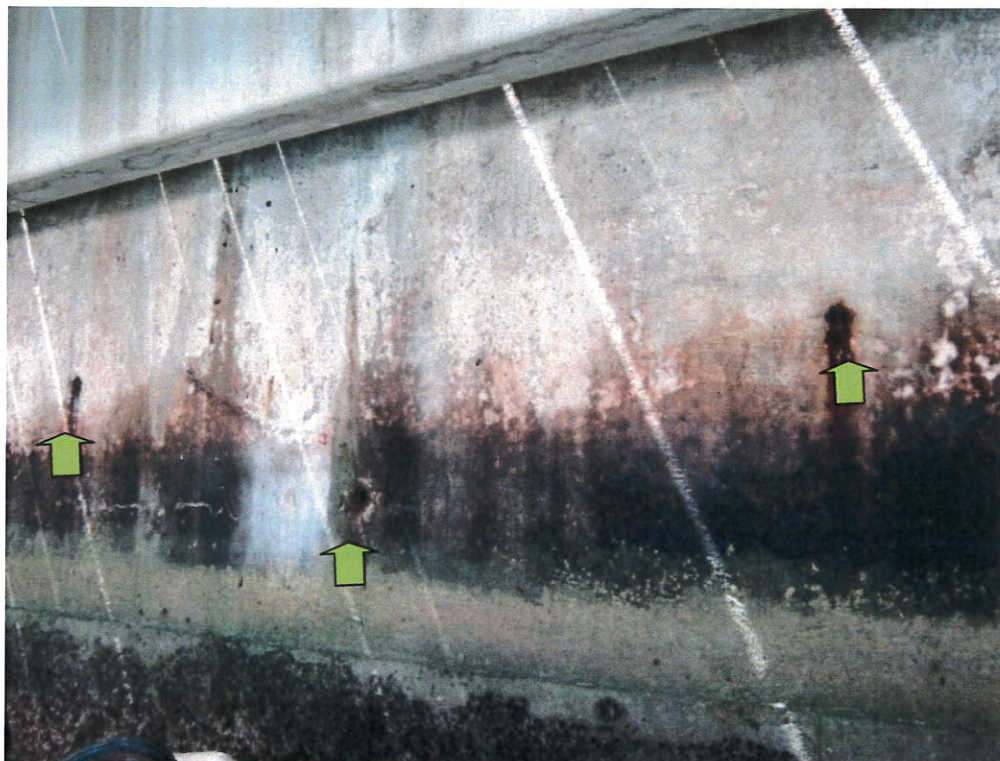
Photo 33: Corroded steel rods noted over the length of wall.
