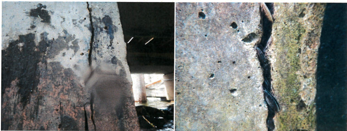
Photo 46: Pier G: couple of 18-inch x 18-inch piles exhibited up to 1/4-inch cracks.
