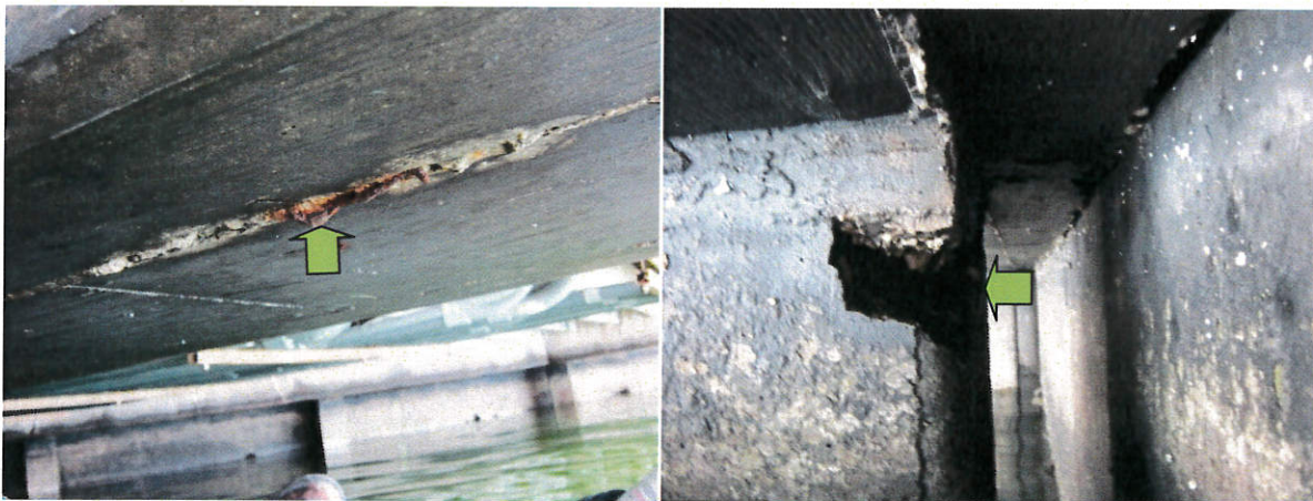
Photo 30: Exposed metal chair at underside of beam (left photo), concrete void and exposed reinforcing at top of concrete pile (right photo - northwest corner area).
