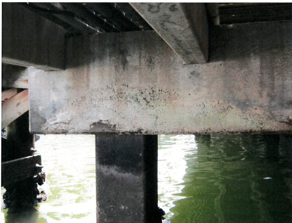
Photo 32: Random honeycombing on pile caps through Entire boardwalk.
