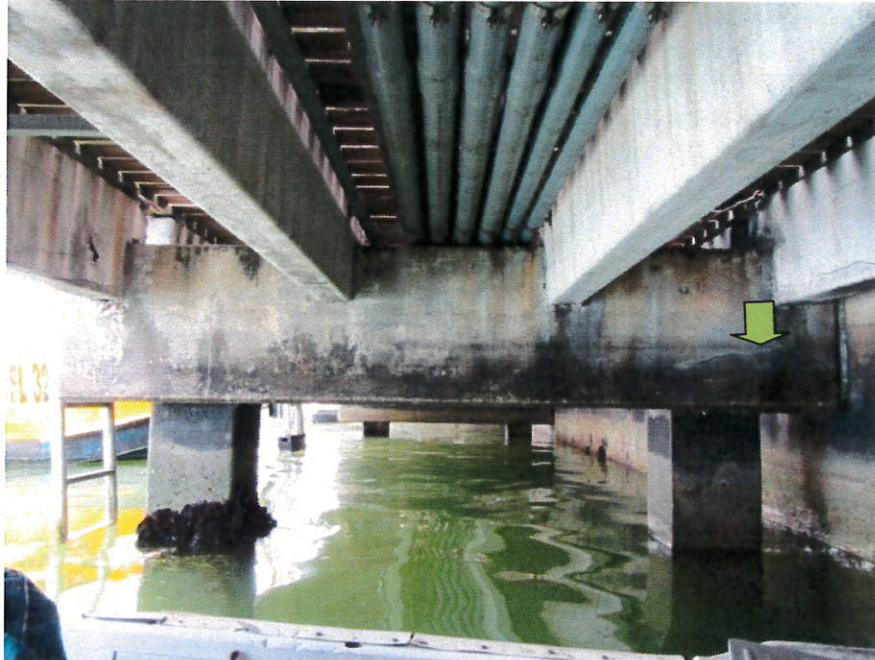
Photo 19: 24x24 concrete pile cap exhibited hairline crack and random honeycombs.
