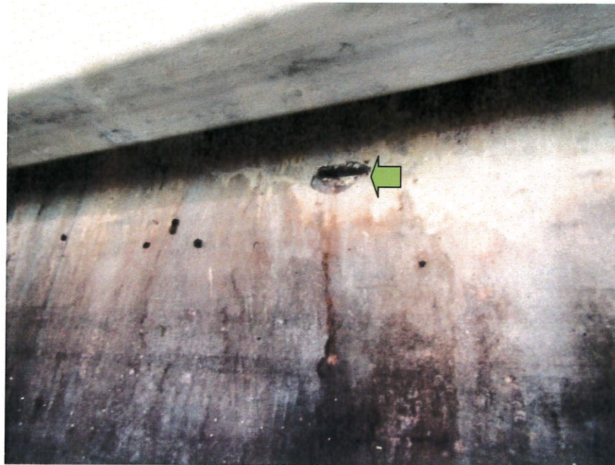
Photo 18: Underside of wood decking; bulkhead above. The waterline, exposed reinforcing noted.
