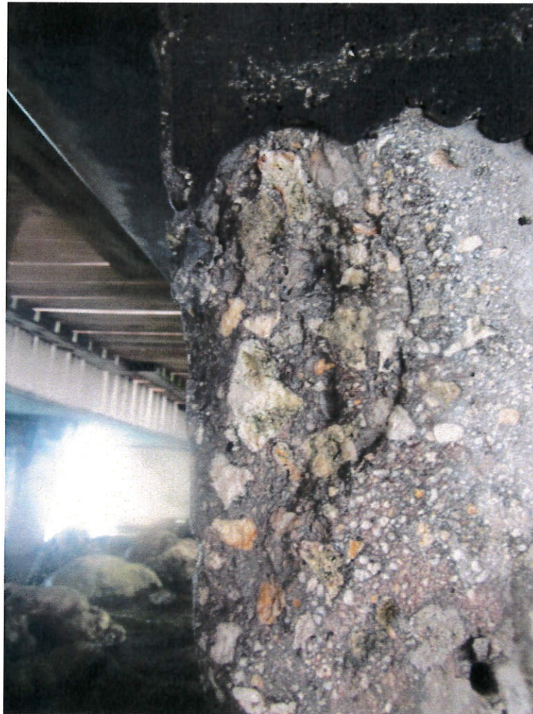
Photo 49: Pier G: Rough concrete surface worn.
