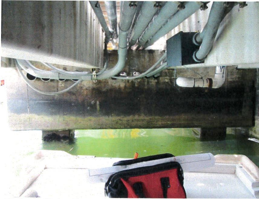
Photo 17: Underside at end of existing construction (wood decking and pre-cast concrete joists); this face of pile cap (Sta 0+00 looking south). Utility chase under wood decking from pile cap to pile cap.
