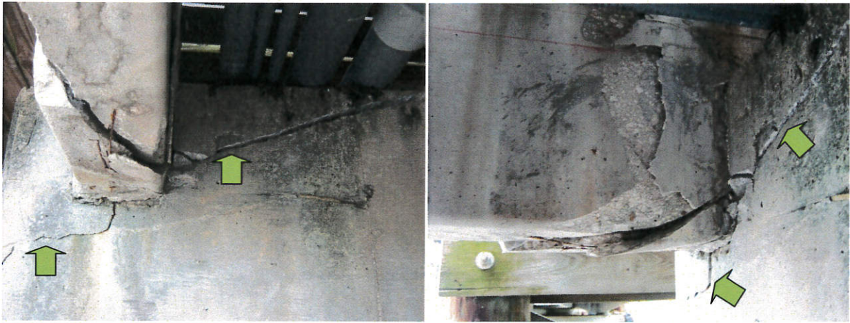
Photo 39: Top corner of pile cap failed (left). Precast concrete joist failed (right).
