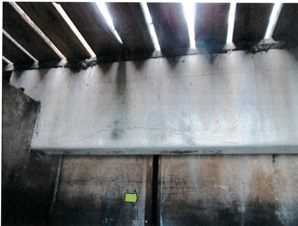
Photo 22: Vertical hairline crack parallel to expansion joint.
