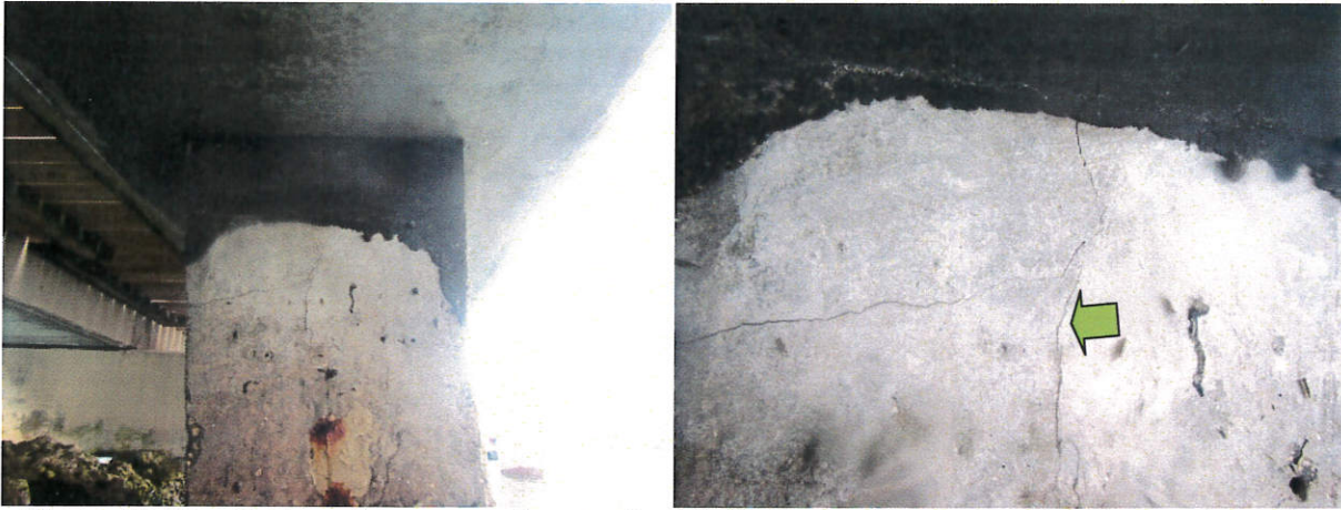
Photo 48: Pier G: sign of concrete piles repaired (left). Same pile, random hairline cracks at the top portion of concrete pile.
