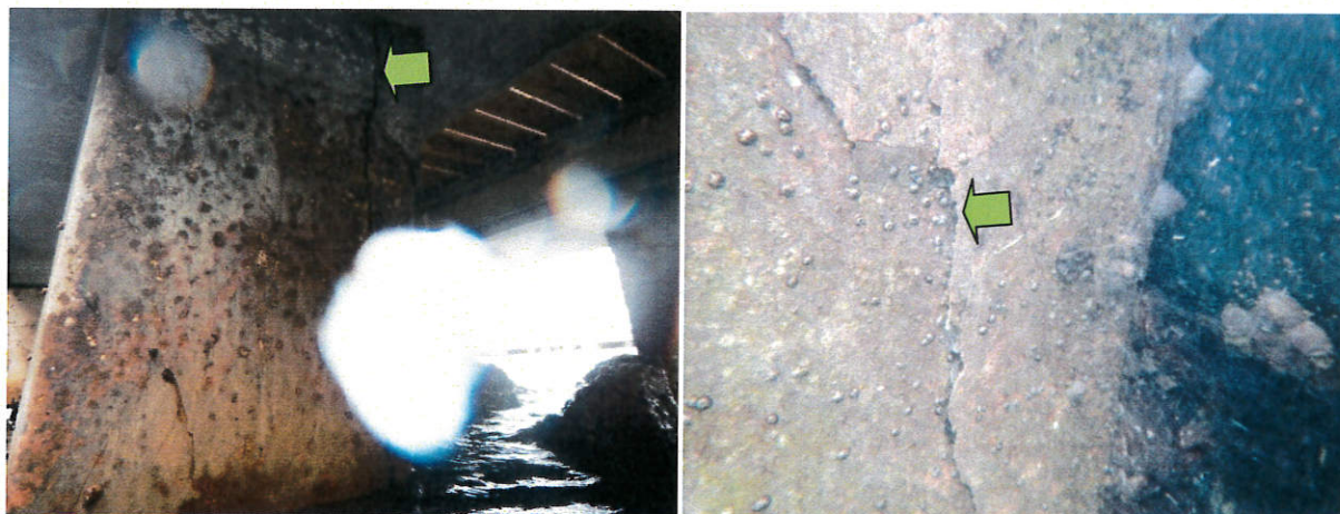
Photo 47: Pier G: couple of 18-inch x 18-inch piles exhibited up to 1/4-inch cracks.
