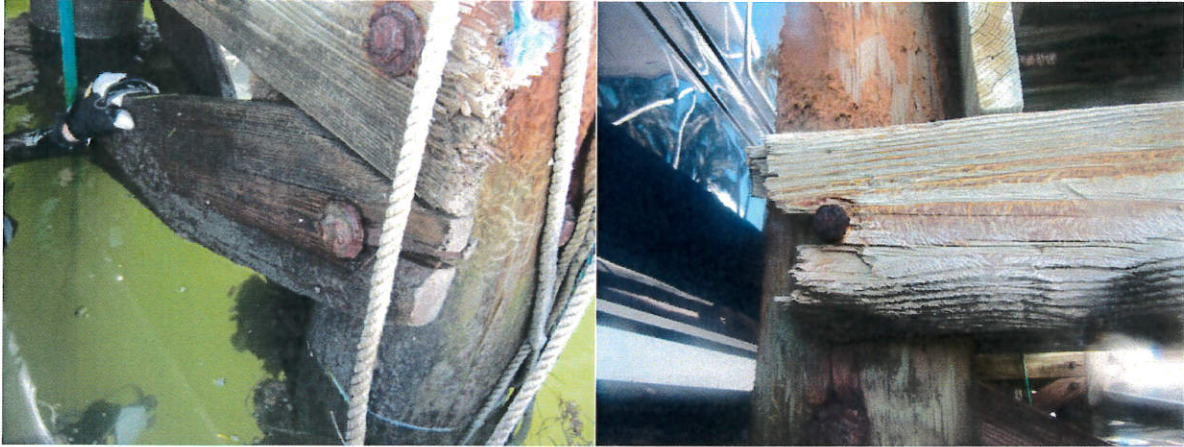
Photo 43: Corroded steel connection corroded and splinted cross bracing (left), horizontal brazing connection failed (right).
