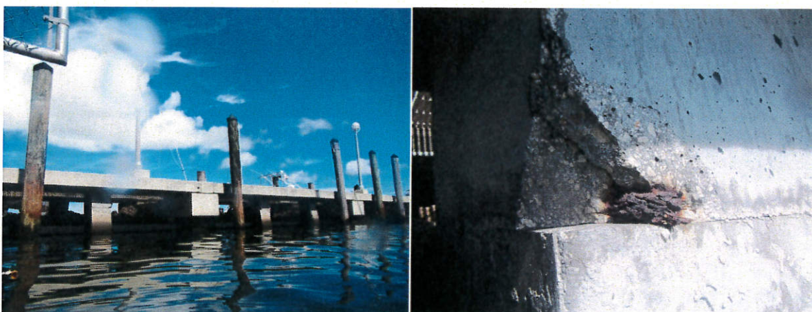
Photo 55: North Concrete Finger Pier (left). Minor concrete deterioration on few piles (right).
