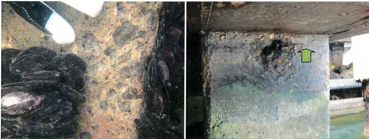
Photo 40: Below water line signs of abrasion (left). Horizontal hairline crack at top of concrete pile (right).
