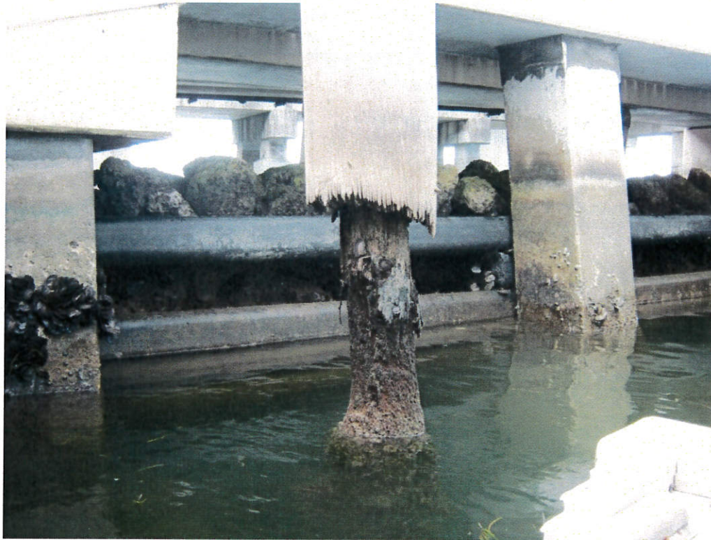
Photo 41: Northeast corner (Pier G) timber pile Deterioration 50% cross section loss.
