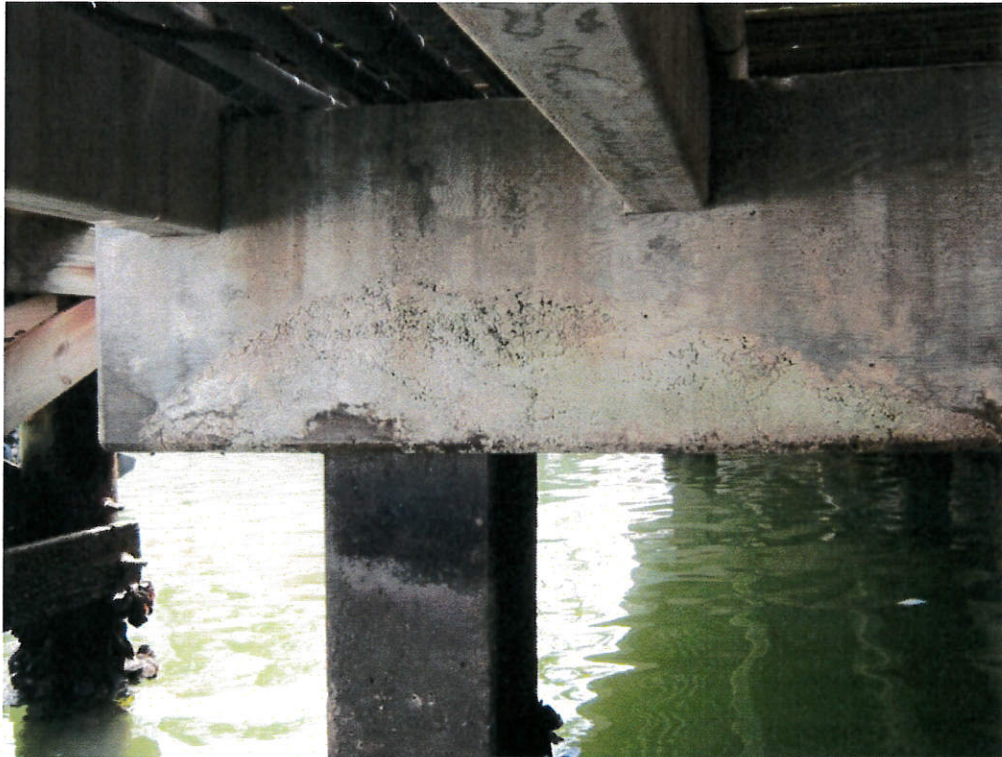
Photo 32: Random honeycombing on pile caps through Entire boardwalk.
