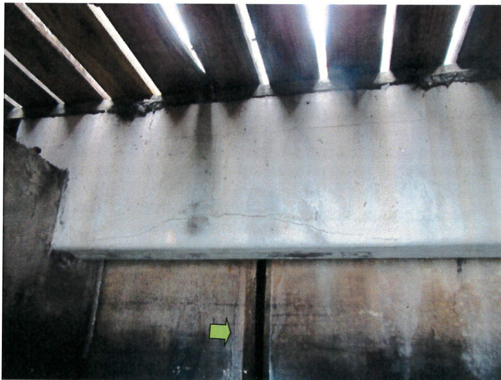
Photo 22: Vertical hairline crack parallel to expansion joint.
