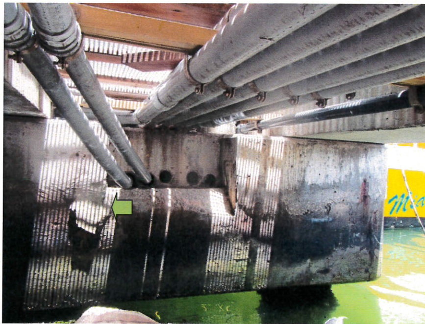
Photo 16: Underside at end of new construction (concrete beams); existing pile cap exhibited minor delamination, sign of previous repairs, corrosion stains, and hairline cracks (looking north). See photo #17 for reference.
