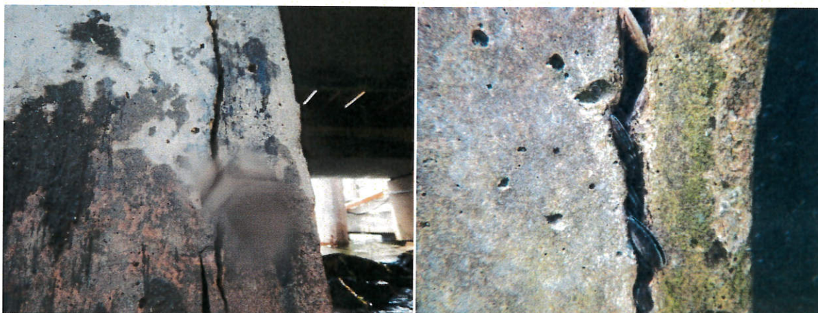
Photo 46: Pier G: couple of 18-inch x 18-inch piles exhibited up to 1/4-inch cracks.
