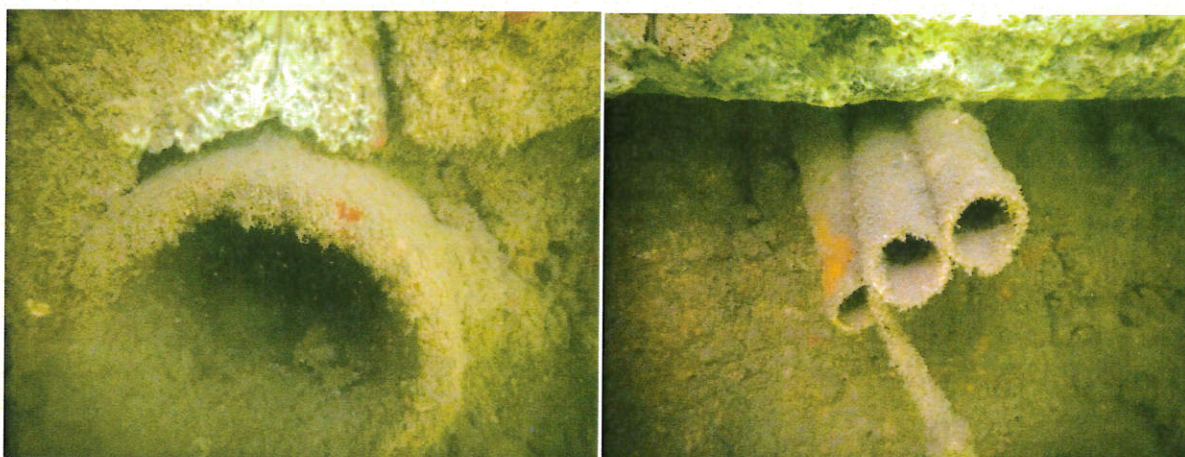
Photo 54: Abandoned outfall and electrical conduits at bulkhead.
