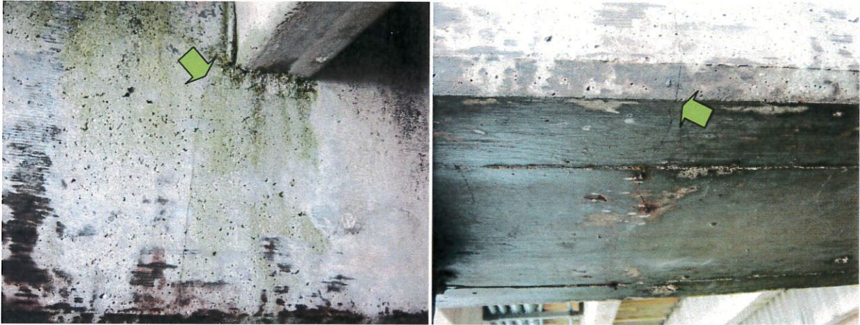
Photo 35: Vertical hairline crack to underside of pile cap.
