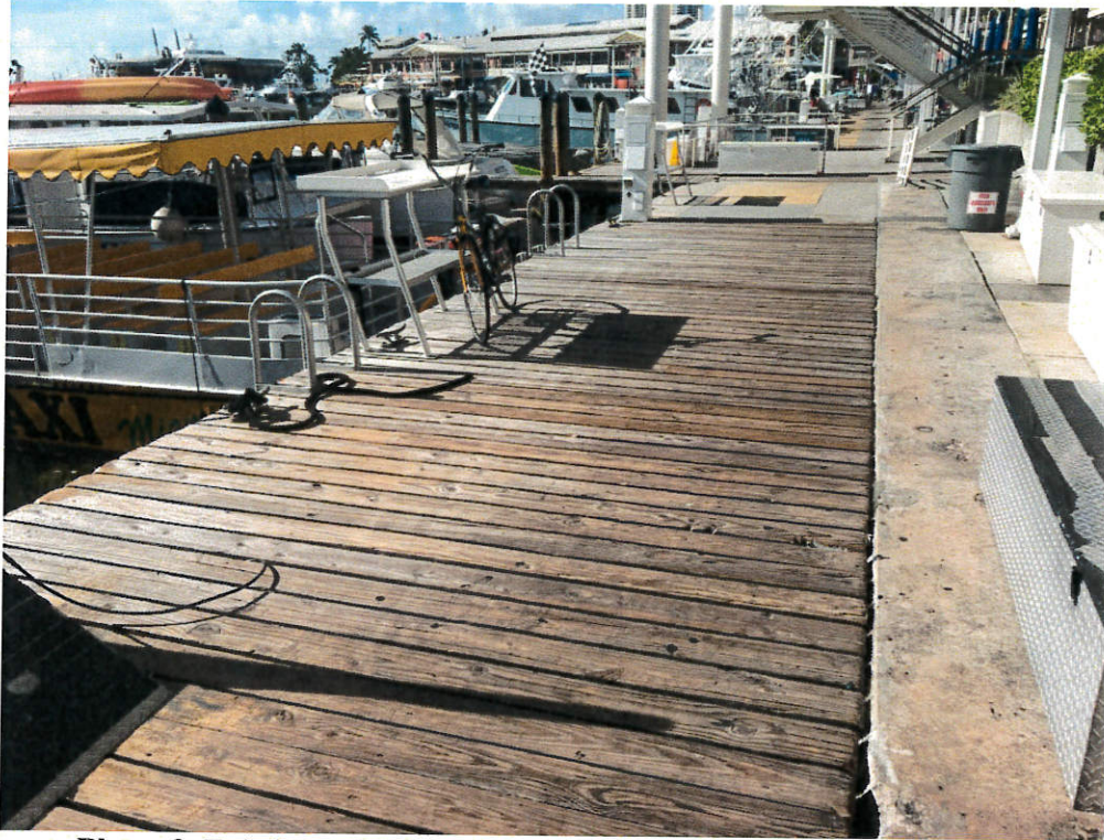
Photo 3: Existing wood decking construction, floating ladder, cleaning station, and pedestals (looking south).
