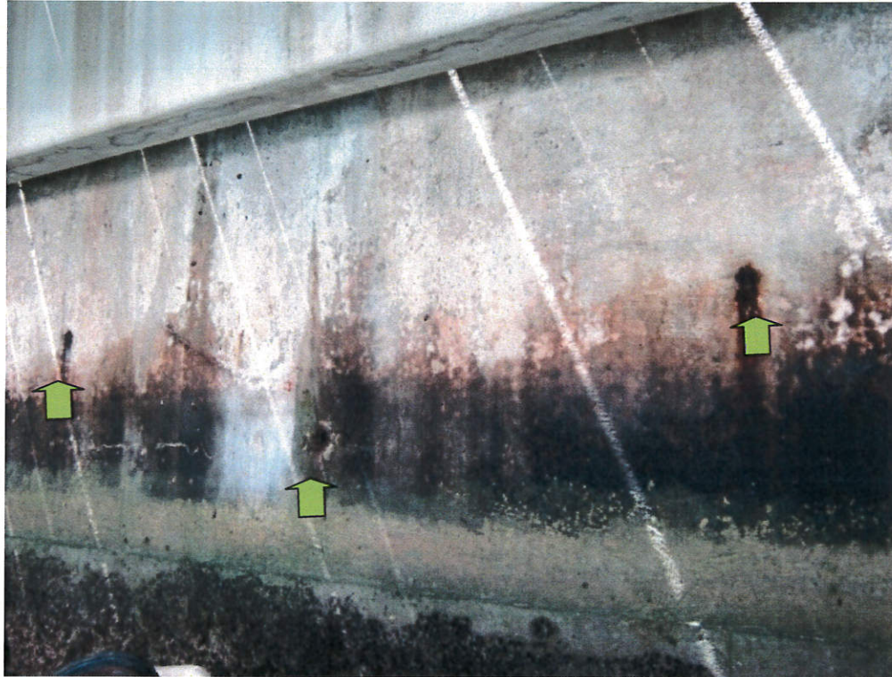
Photo 33: Corroded steel rods noted over the length of wall.
